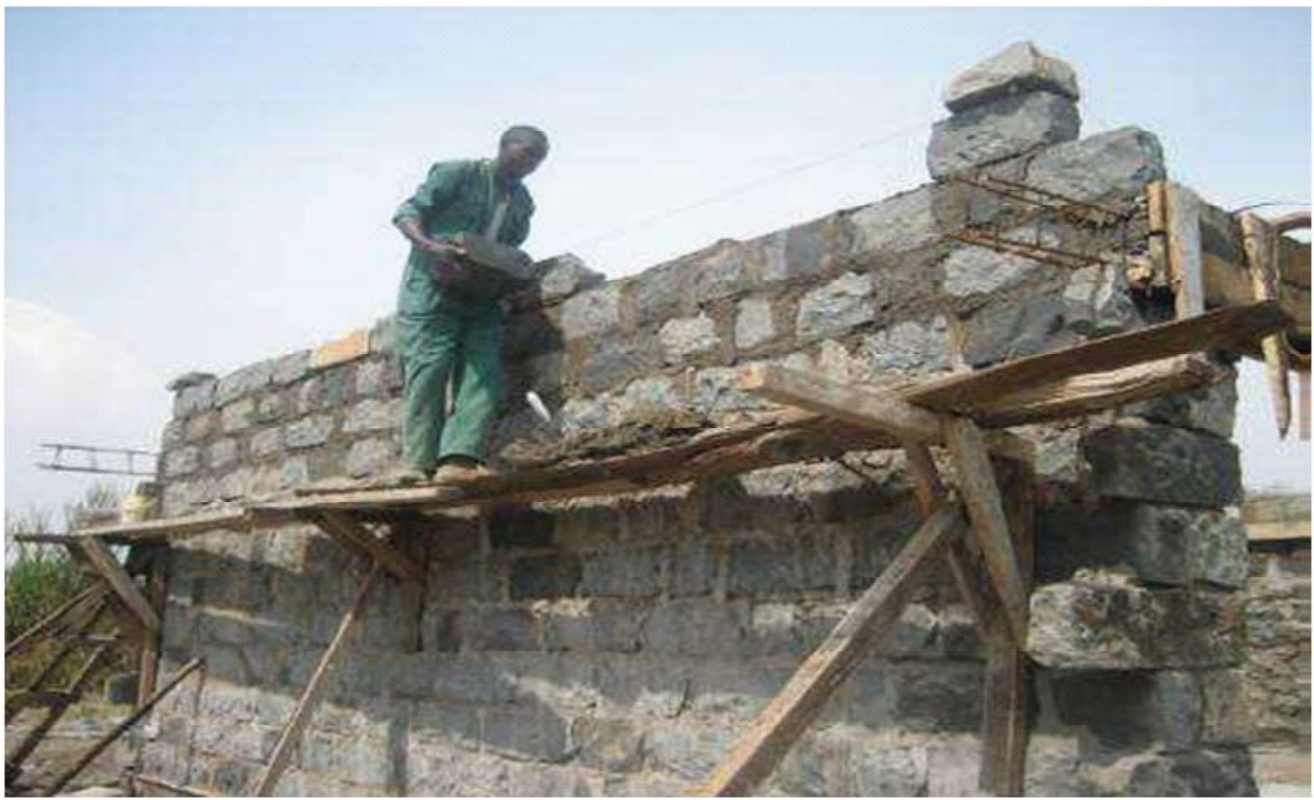
CONSTRUCTION OF THE NURSERY CLASSROOM FUNDED BY THE DEPOSIT PROTECTION FUND BOARD AT THE KAJIADO CHILDREN'S HOME IN PROGRESS.
